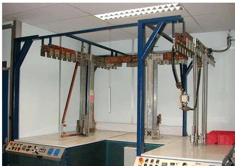
Temperature rise test station rated 4000 A
